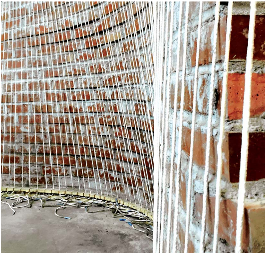
Figure 5. Ruled surface brick wall prototype and string formwork secured at curved base.
